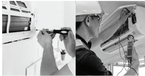
Complicated Wiring Steps Difficult Connecting
